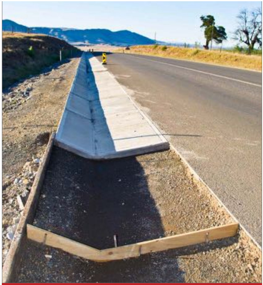
New V-drains are installed on the R56 to enhance safe and efficient surface water run-off
