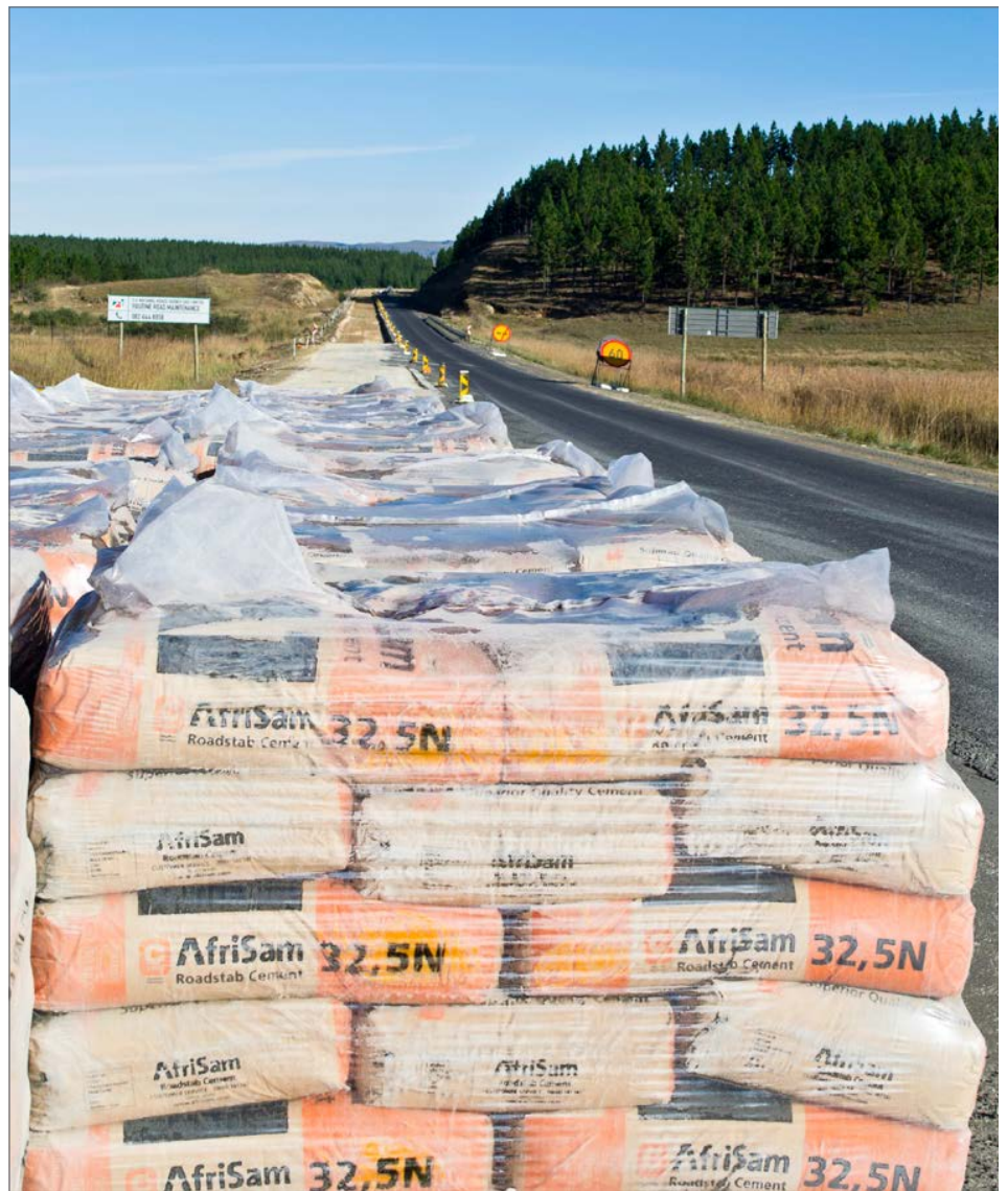
AfriSam's Roadstab is a specially formulated composite cement and is being used by Tau Pele on its R56 contract in the Eastern Cape
