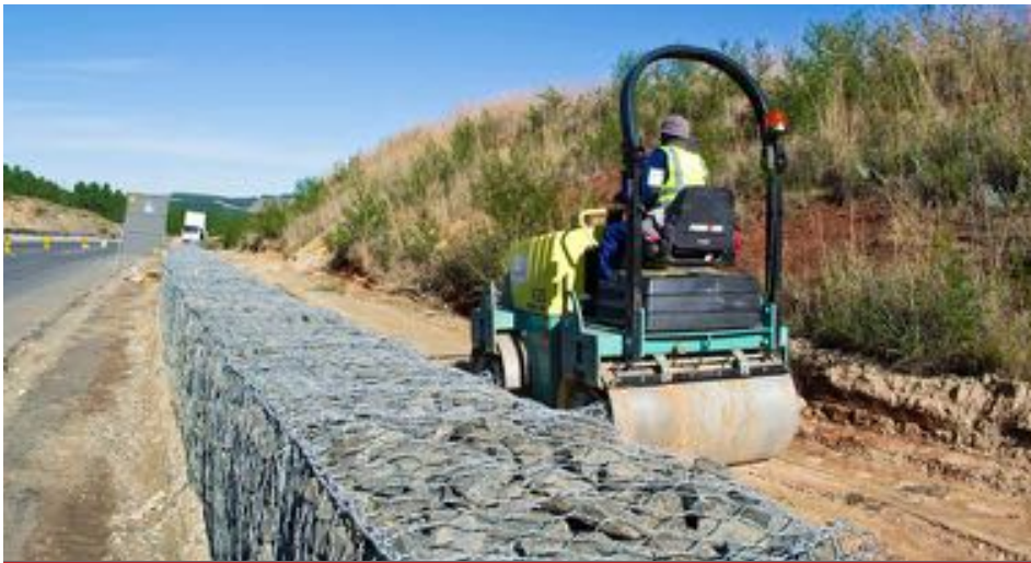
Compacting ground between the newly installed gabion and a soft cutting on the R56, before placement of backfill
